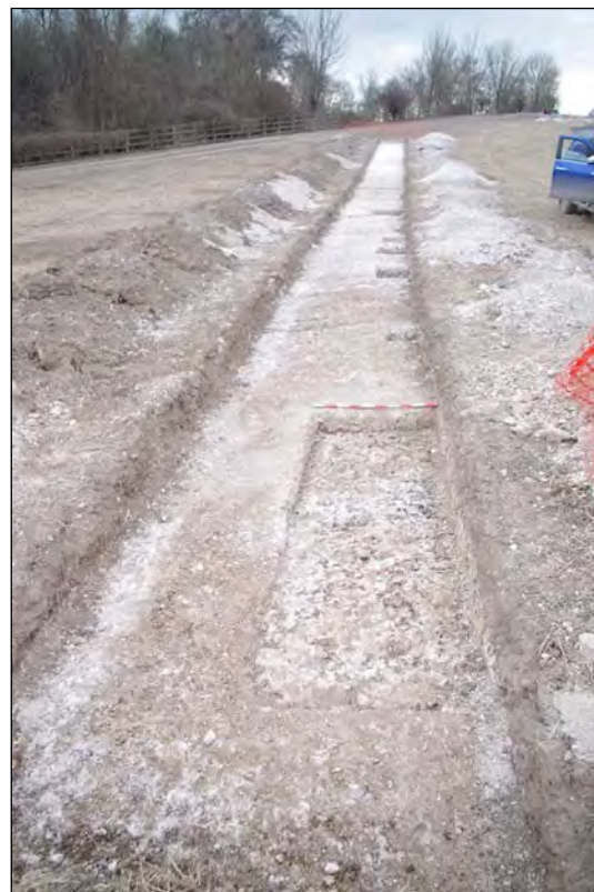
Plate 12.10: View from the north-east of shallow cut 50905 truncating the chalk (excavated in hand-dug slots)
